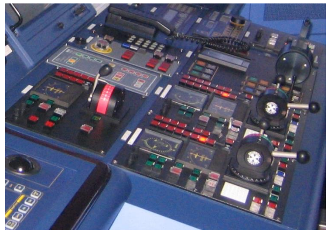
Figure 3b: DP Thruster Control Panel
